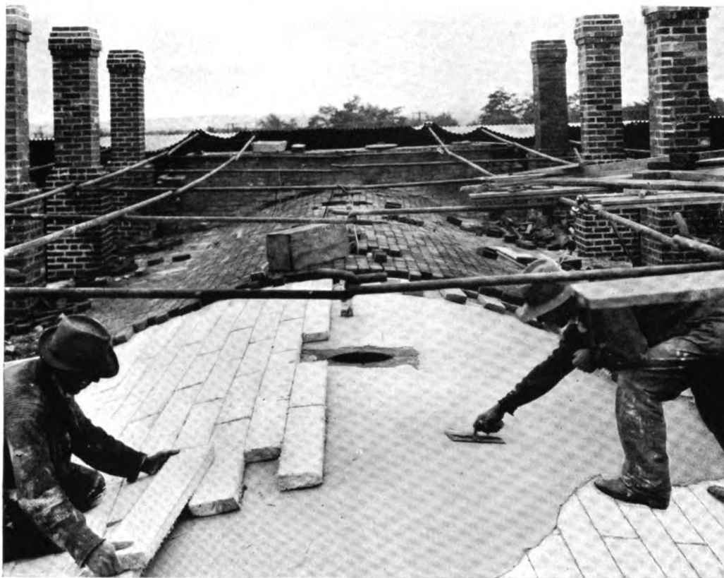
Applying Superex Blocks to top of rectangular down-draft kiln at Hazelton Brick Co., Hazelton, Pa.
