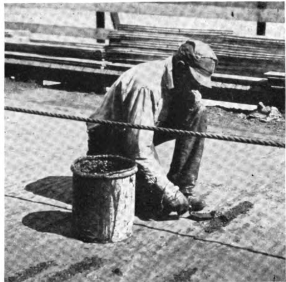
Patching holes in sub-floor with cold patch material before laying Asphalt Bridge Plank
