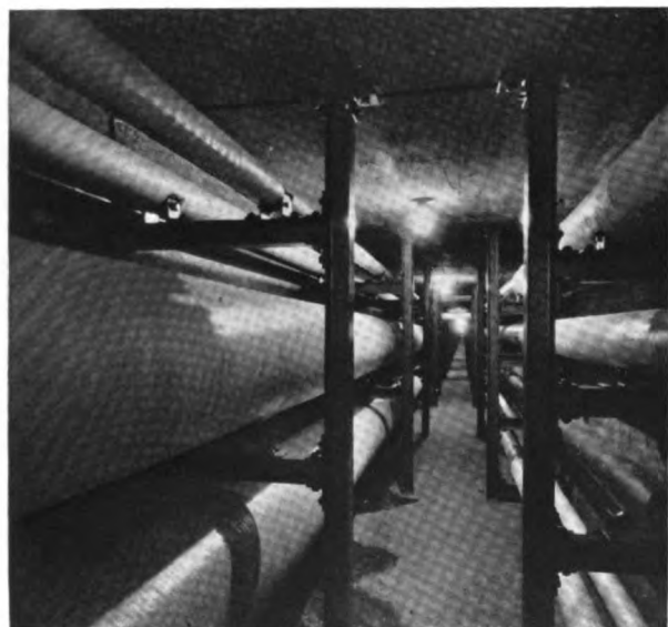
J-M Wool Felt on lines in walking tunnel. United Aircraft & Transport Corp., East Hartford, Conn.
