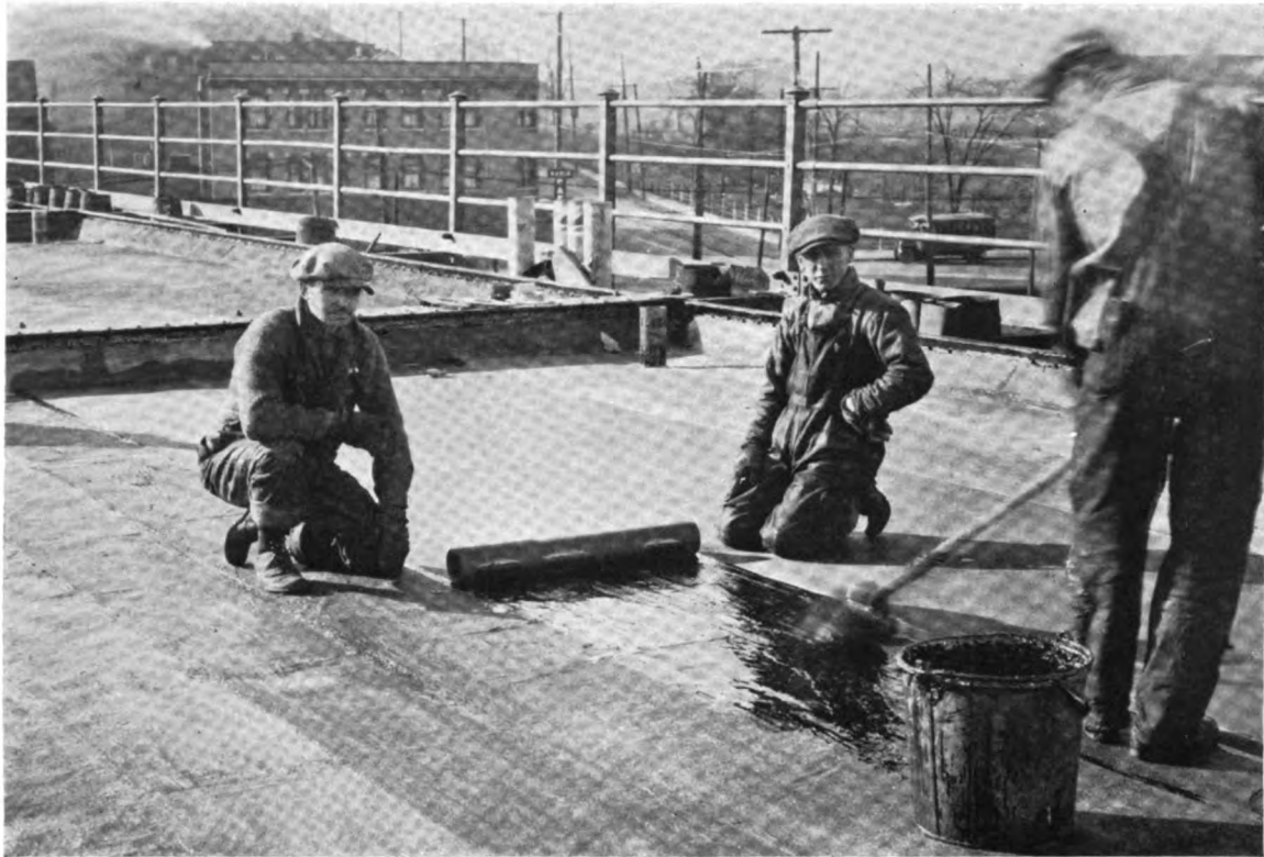
J-M Waterproofing on the Niagara River bridge of the Michigan Central R.R.
