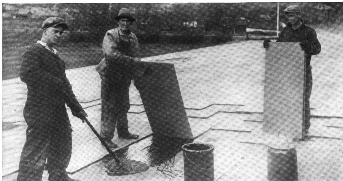
Three layers of ½" J-M Rigid Roofinsul, to be overlaid with a J-M Built-up Roof
