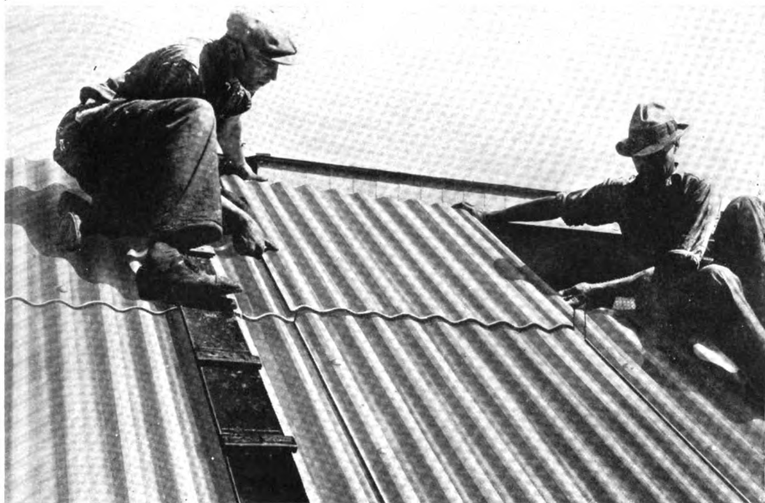
Laying J-M Corrugated Transite Roofing. The cut corner construction permits a tight joint with straight lap lines, and results in a durable, attractive roof
