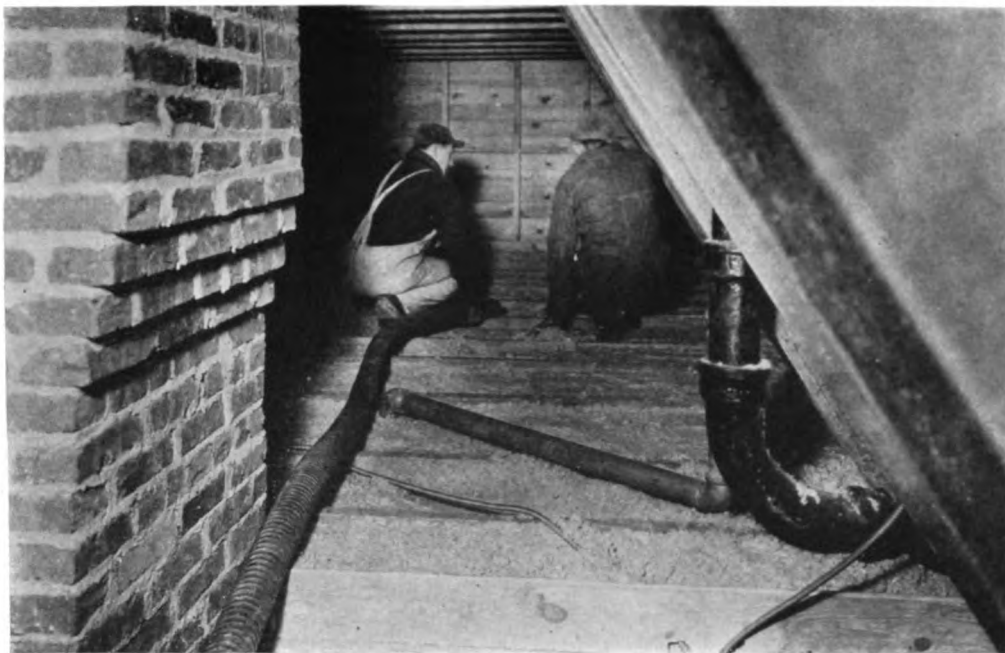
Filling in between the joists of an unfloored attic with J-M Home Insulation, insures warm rooms below
