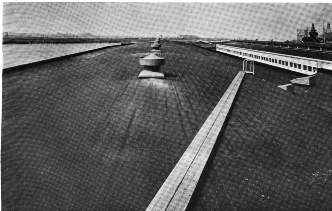
J-M Super Class A Built-up Roofs on the Grove St. docks, Port of Oakland, Calif.
