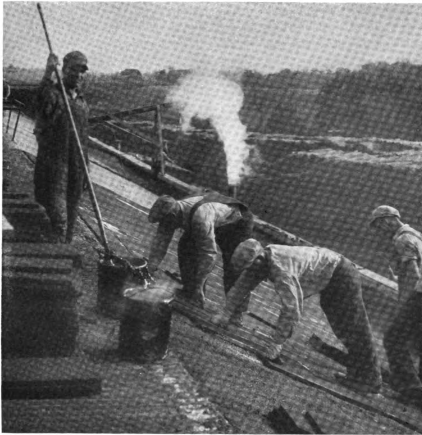
J-M Insulated Rot-proof Roof over machine room, Combined Locks Paper Co., Combined Locks, Wisc.
