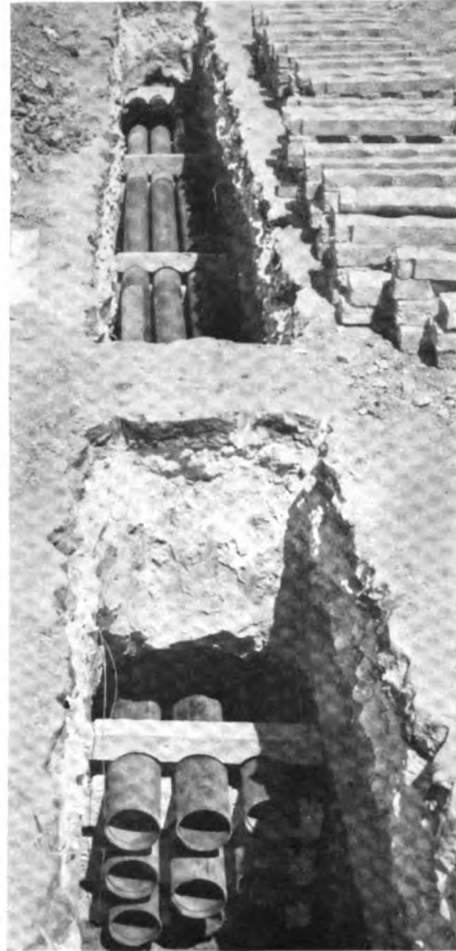
Intact sections of pavement and base serve as braces for top of ditch. Conduit installation by Los Angeles Gas and Electric Corp., Los Angeles, Calif.
