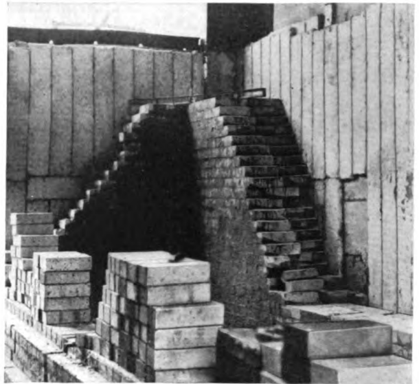
Superex Combination Insulation, 3 1/2" thick, between Transite casing and fire brick lining of Gyro tube still
