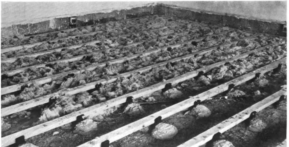
In fireproof apartment sound-isolation construction, J-M floor chairs are grouted in with cement. Sound isolation fill is placed between the stringers
