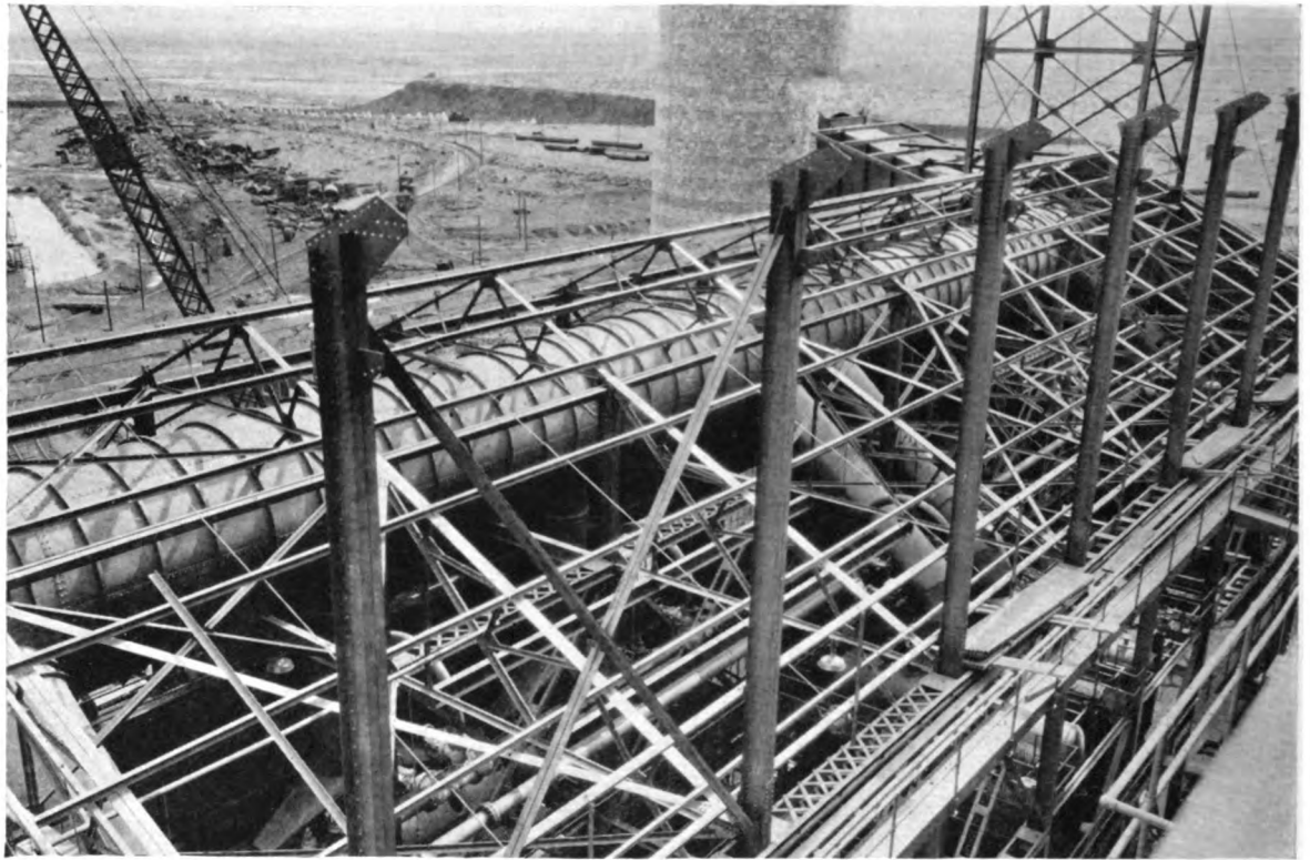
Boiler up-takes and flue to stack at large copper smelter, insulated with Sil-O-Cel Natural Brick and Sil-O-Cel Coarse Grade
