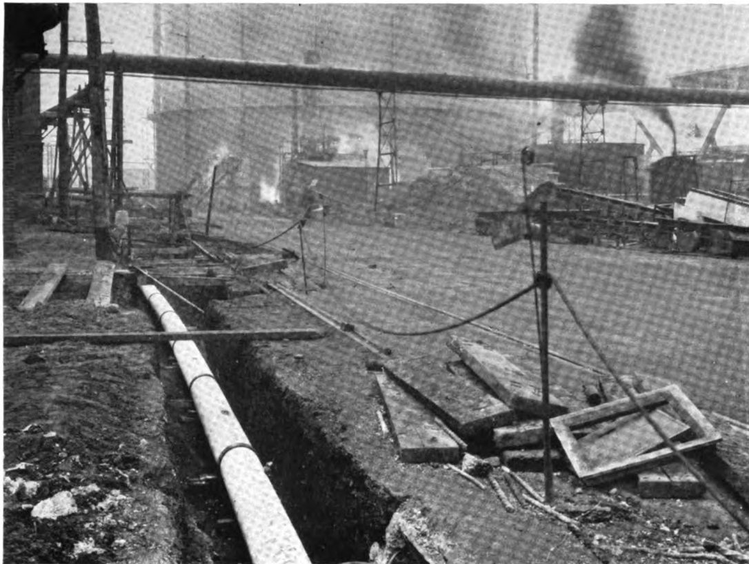
Twelve-inch Class B Transite Pipe for water mains in a large gas plant
