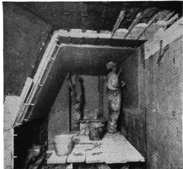
Boiler breeching lined with 2 1/2" Sil-O-Cel Natural Brick and Semi-Refractory Cement
