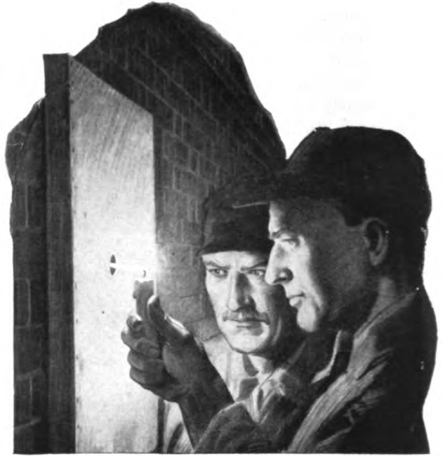
To determine leakage, a square of cardboard, pierced with a small hole and fastened to a wood frame, may be pressed against a boiler wall and the edges temporarily sealed. The inrush of air through the hole shows the leakage.
