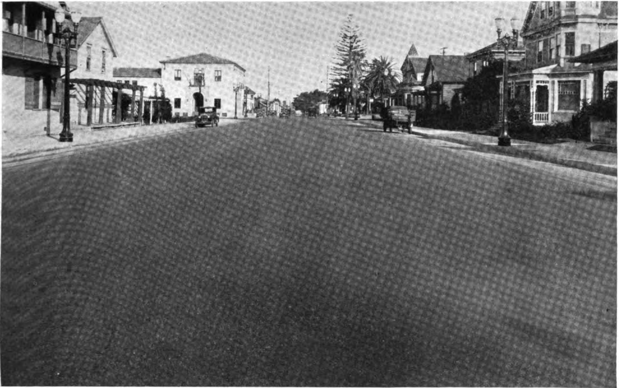
Fig. 1. Celite used with excellent results in asphalt paving on Chapala Street, Santa Barbara, Calif. Richardson Construction Co., Santa Barbara, Calif., Contractors
