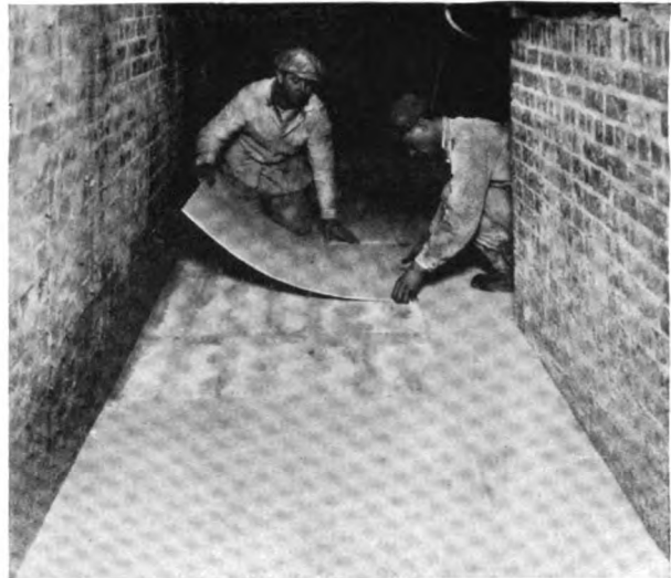
Laying J-M Millboard over Superex blocks between side walls and brick pier in base of asphalt still
