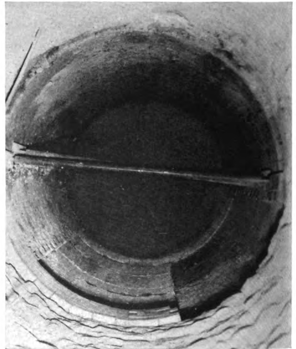
Superex insulation in rotary kiln, showing longitudinal timber and cross-jack method of installation
