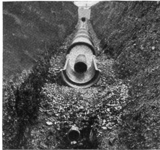
In the J-M System the conduit is completely filled with asbestos fibre, and adequate drainage provided by bell and spigot pipe in broken stone
