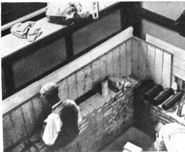
Superex Combination Insulation, 3 1/2" thick, applied between Transite casing and fire brick in Gyro Process Tube Still
