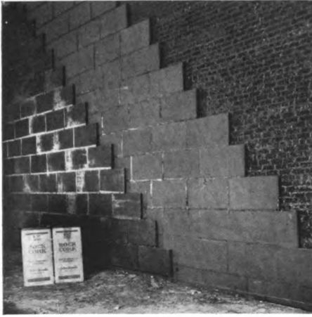
Installation of Rock Cork Sheets in the Miller Brewing Company, at Milwaukee, Wisconsin. A total of 150,000 board feet of this insulating material was used in this one installation.
