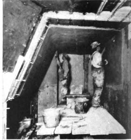
Boiler breeching being lined with two-and-one-half inches of insulating brick and a facing of semi-refractory cement.
