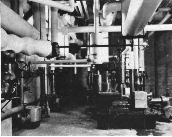
Johns-Manville 85% Magnesia Pipe Insulation installed on the steam lines in the power plant of the Elmira, N. Y., State Penitentiary.
