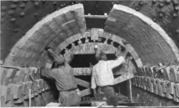
Left: Rotary cement kiln being insulated with Superex Blocks between steel shell and refractory lining. Superex Blocks are practically standard insulation for the severe service encountered in lime and cement kilns. Below: Applying Superex Blocks to top of a rectangular kiln for the firing of face brick.
