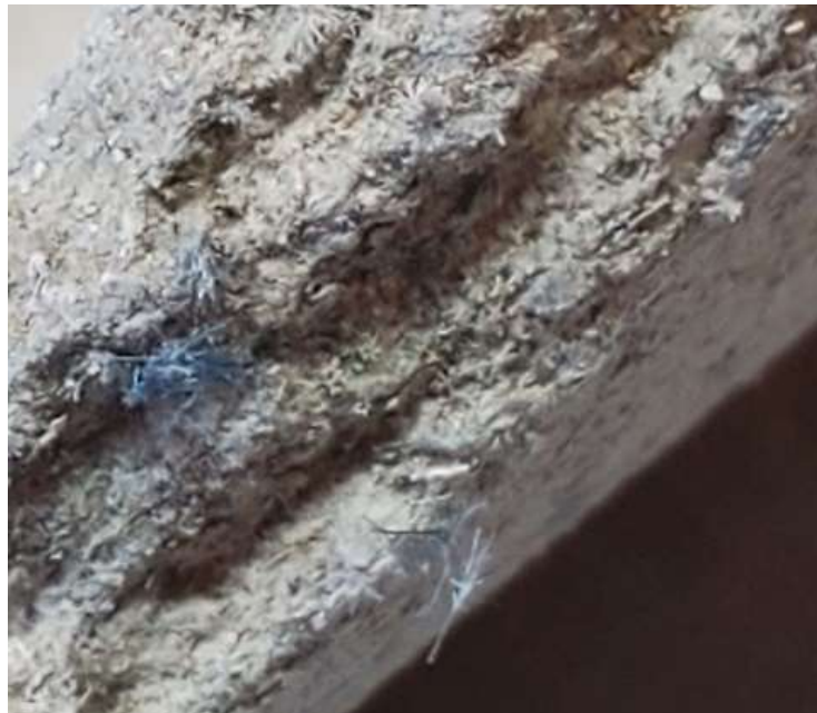
Crocidolite (Blue Asbestos) Fibers being Liberated to the Environment from a Deteriorating Asbestos-Cement Pipe
