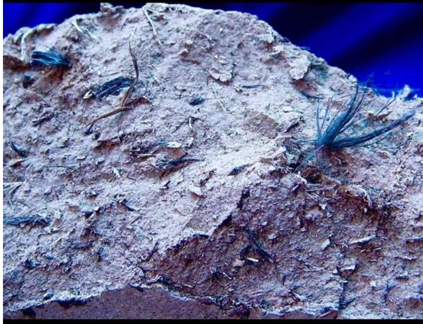
Crocidolite (Blue Asbestos) and Chrysotile (White Asbestos) Fiber Bundles being Liberated to the Environment from a Deteriorating Asbestos-Cement Pipe
